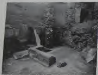
FIG. 16. S. Sebastiano. Ambulatory wall and foundations with fragments of original remains of villa.
